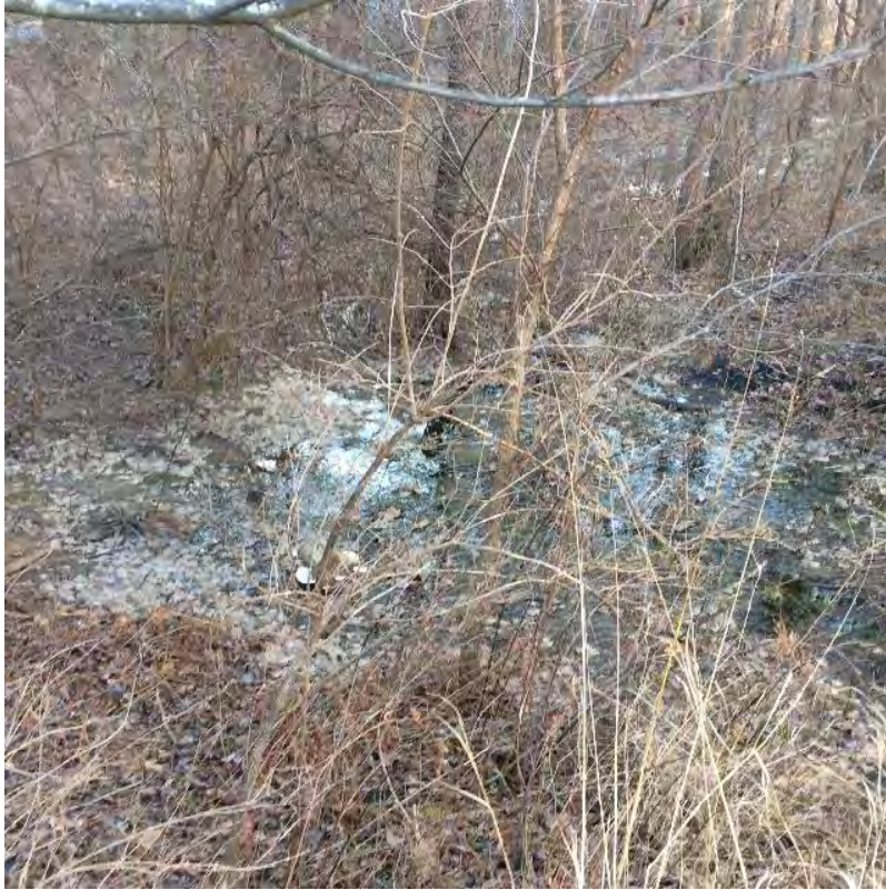
Tree Growth on Embankment
