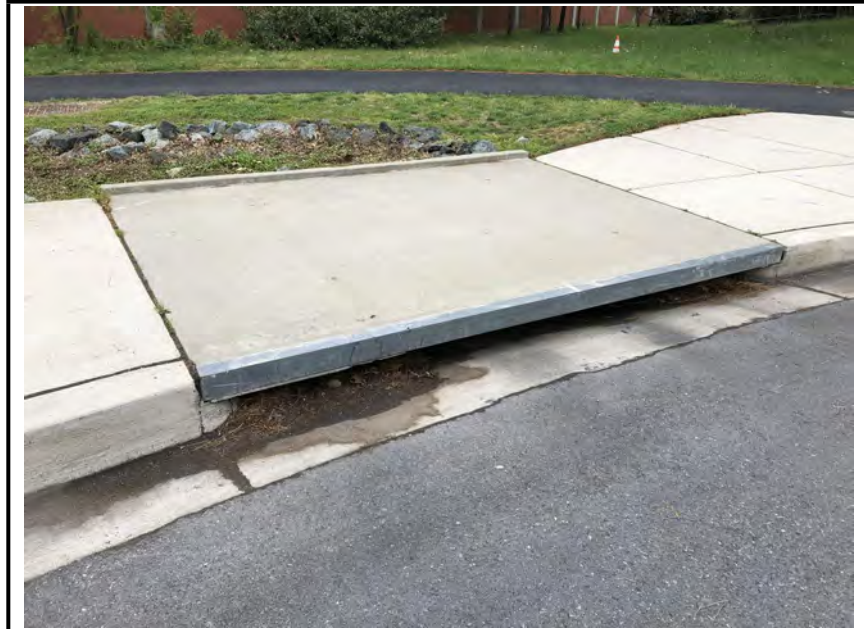
Photo #1: Inflow structure.
