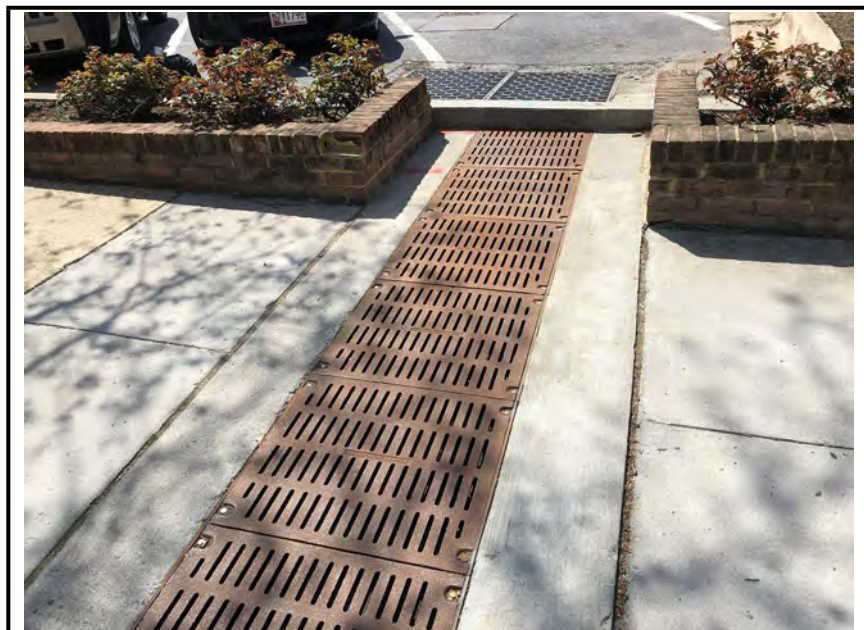
Photo #4: Trench drain that leads to the facility.
