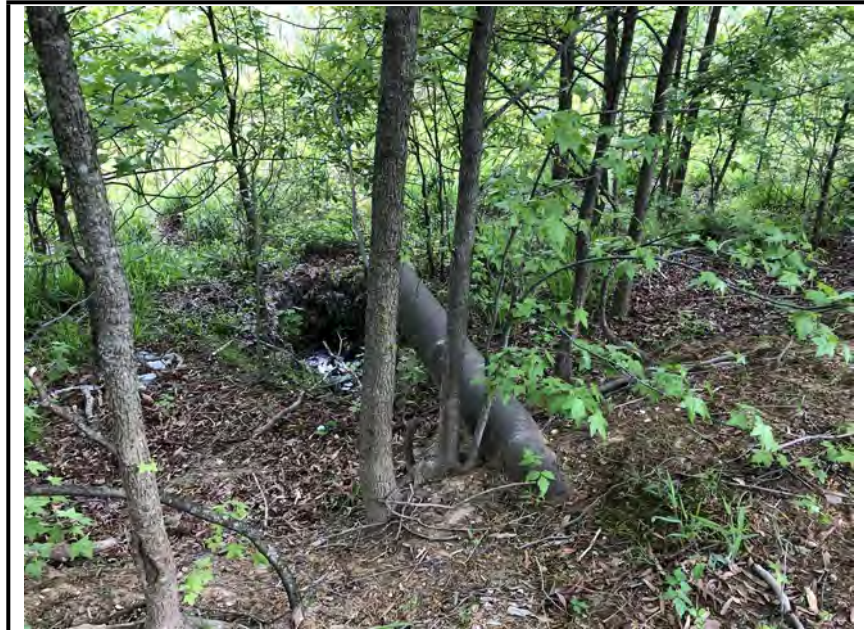
Photo #5: Erosion around inflow pipe.
