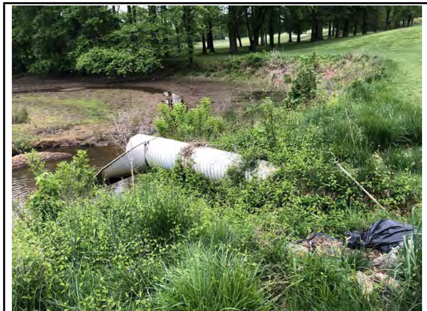
Photo #6: Exposed inflow culvert.
