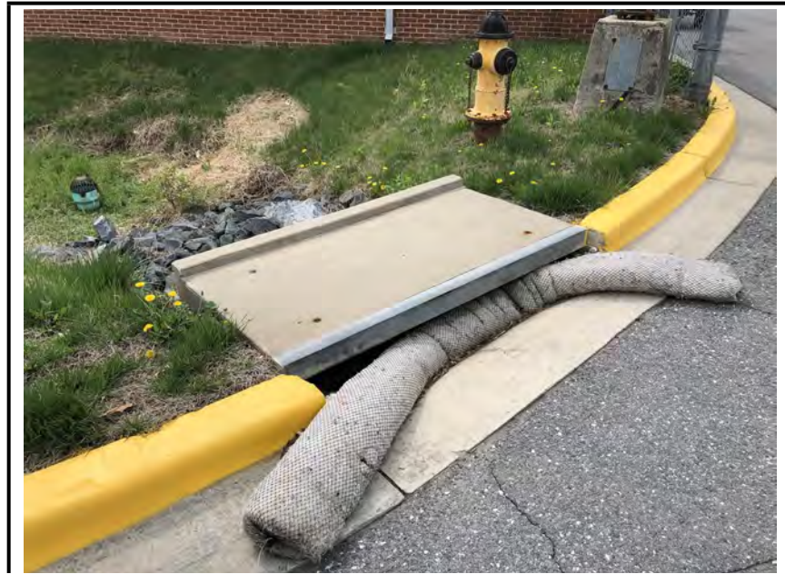
Photo #1: Filter log stuck inside of the inlet.
