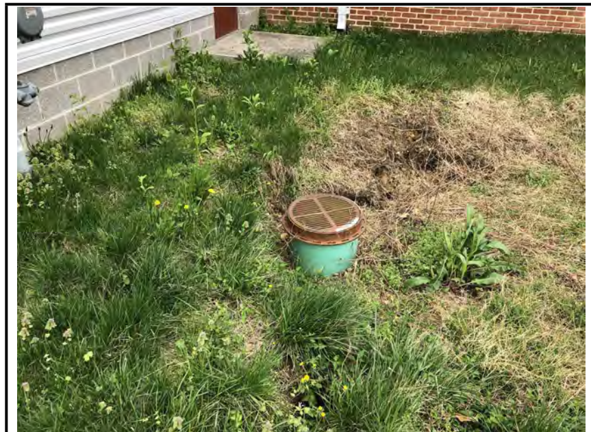
Photo #4: The riser outlet in the facility.
