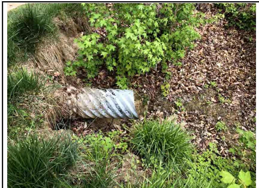
Photo #2: Erosion around inflow pipe.
