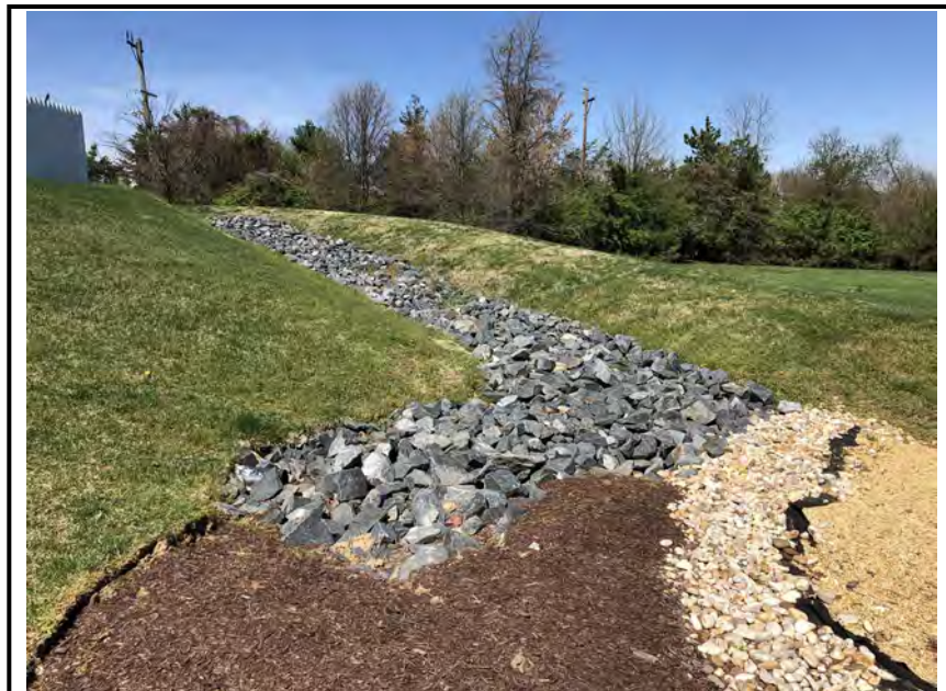
Photo #4: The riprap channel that leads into facility 035. Exposed filter fabric visible.
