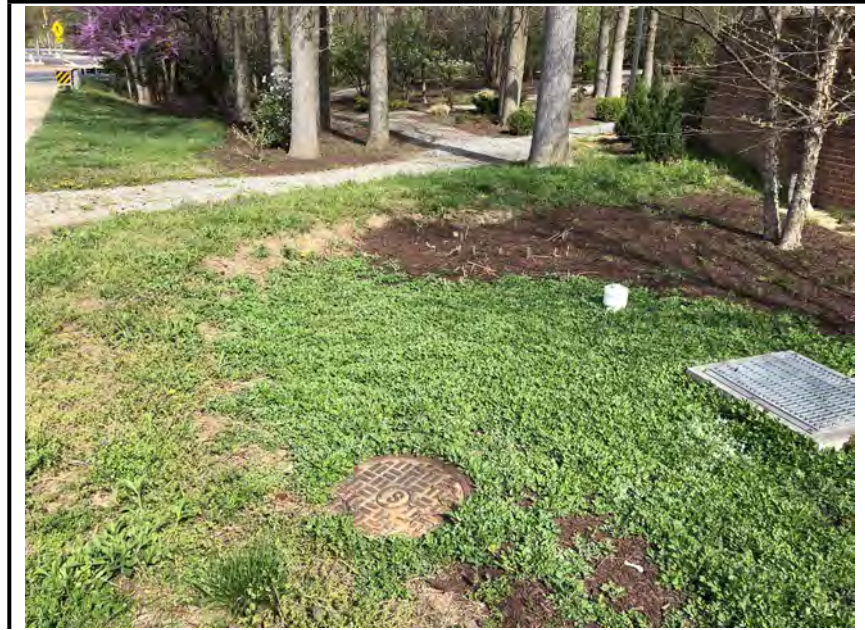
Photo #1: Weeds inside the filter area.
