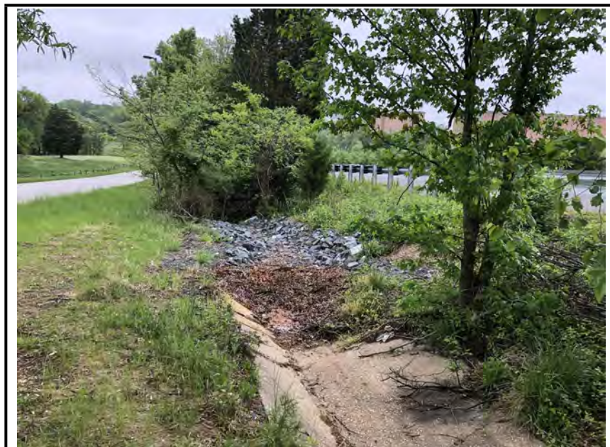
Photo #2: Inflow into the facility.
