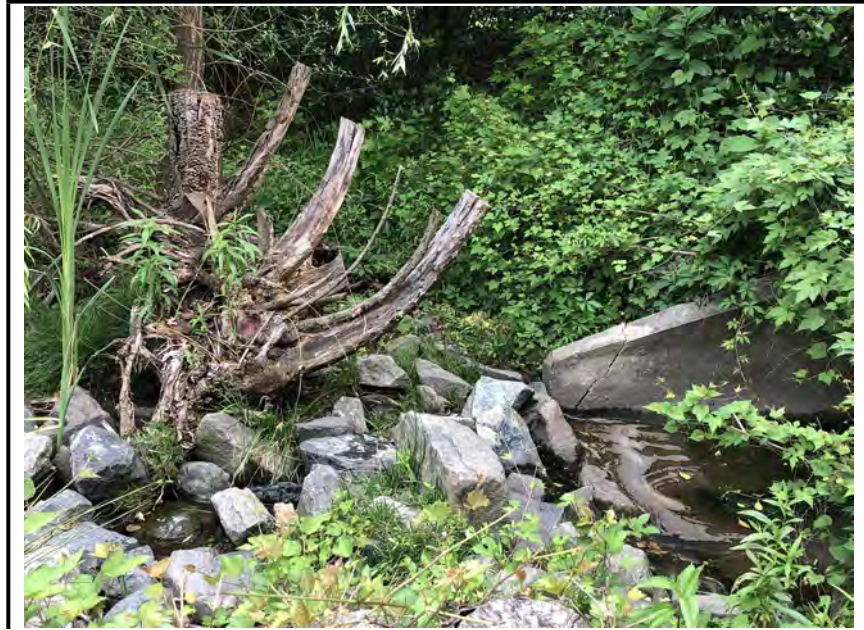
Photo #3: Dead tree stump in front of the culvert inflow point.
