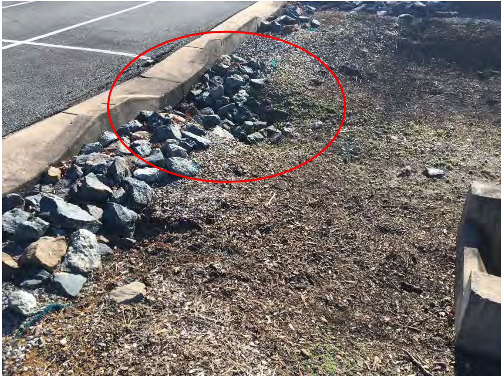
Erosion at inflow, water flows under curbing
