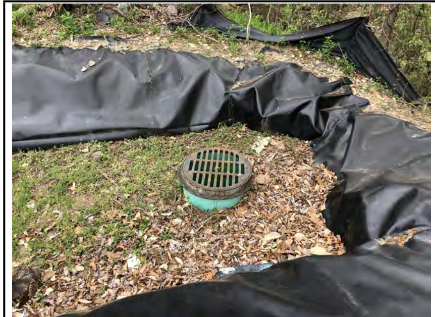
Photo #3: The riser outlet on SWF 22, and erroneous silt fence behind the facility.
