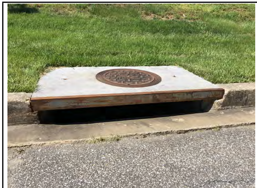
Photo #2: The curb inlet structure that leads into the facility.
