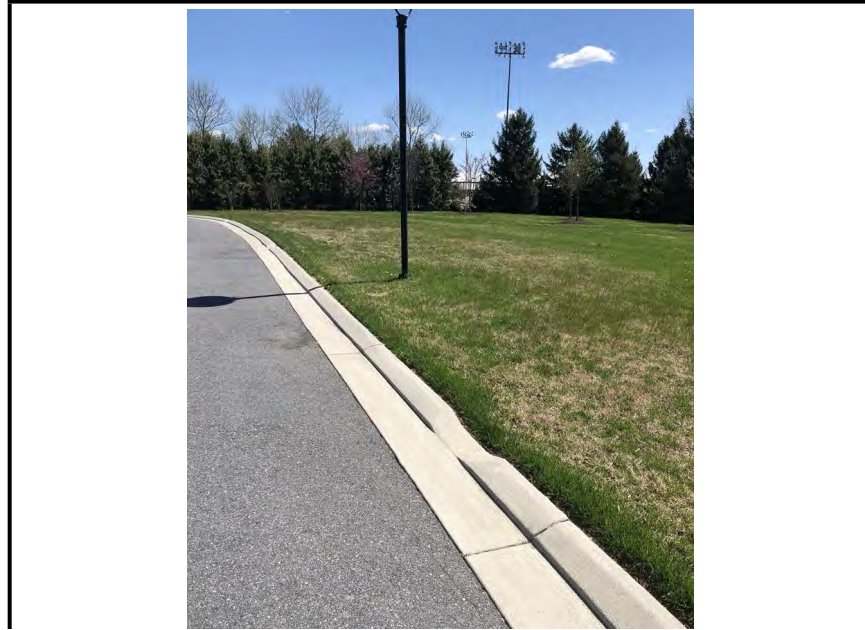
Photo #1: A section of the non-rooftop disconnect area.
