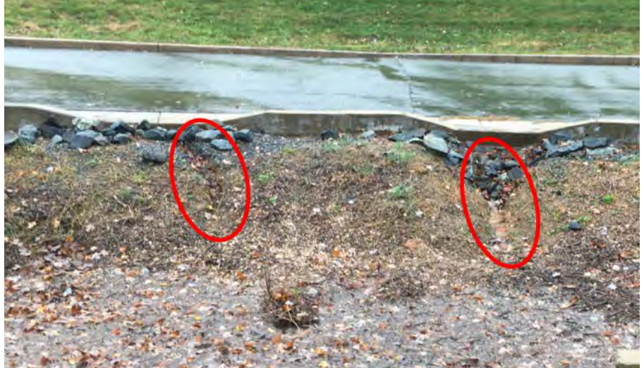
Figure 4 - Existing erosion at side slopes
