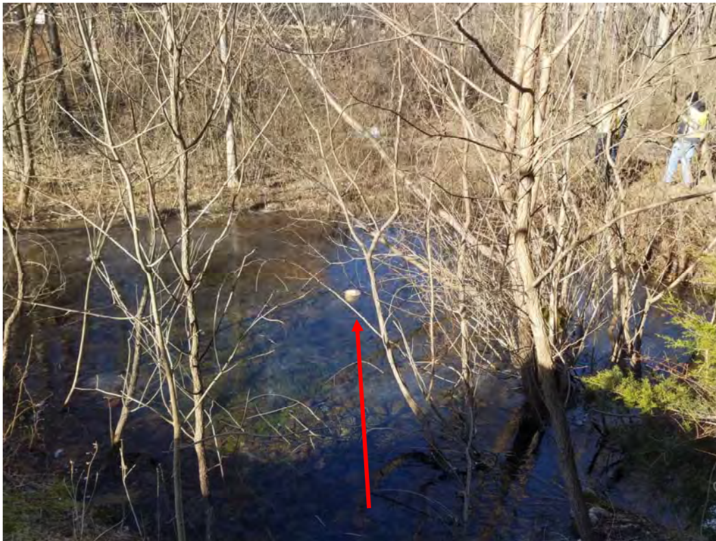
Ponding within BMP, Observation Well submerged, minor reseeding at inflow - sheetflow.
