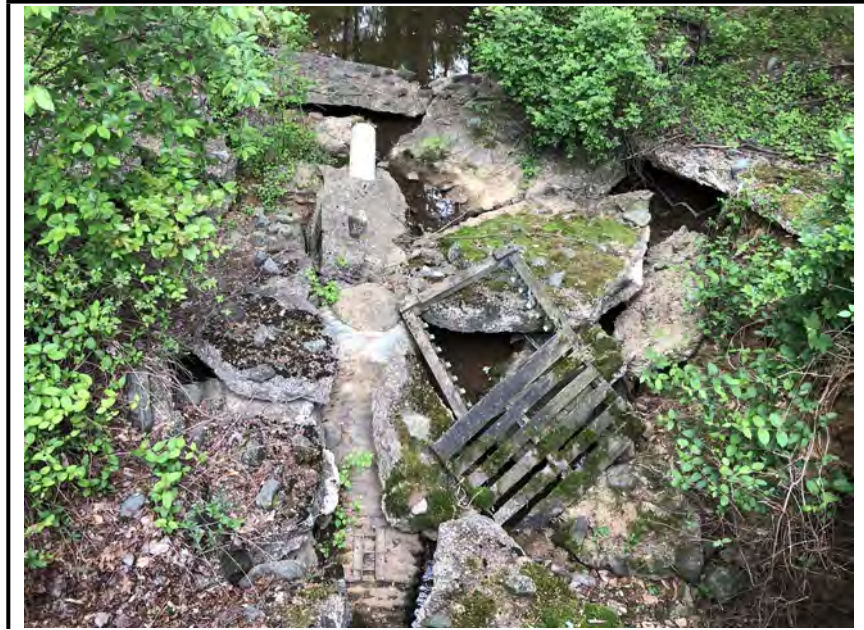
Photo #7: Crumbling dam outflow.
