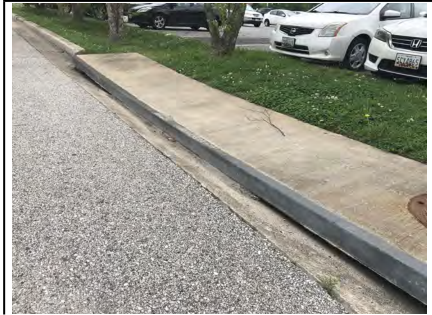
Photo #3: Collapsing curb inlet.
