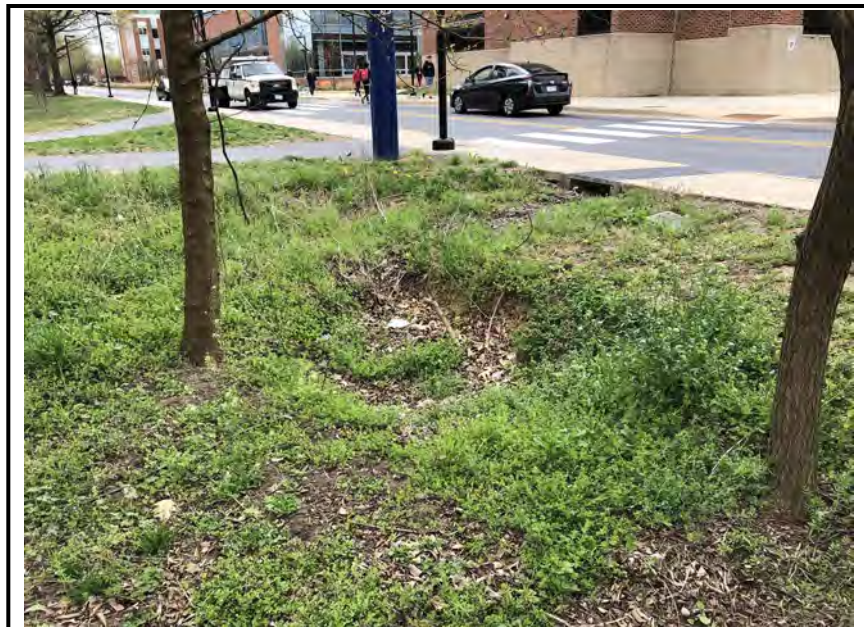
Photo #4: Erosion on the side slopes.
