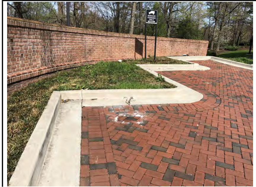
Photo #1: Stains on the pavers.
