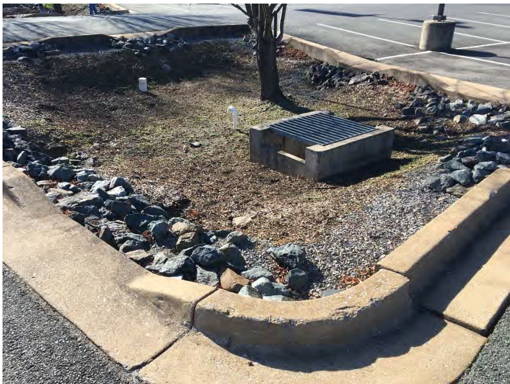
Overall, Overflow Device
