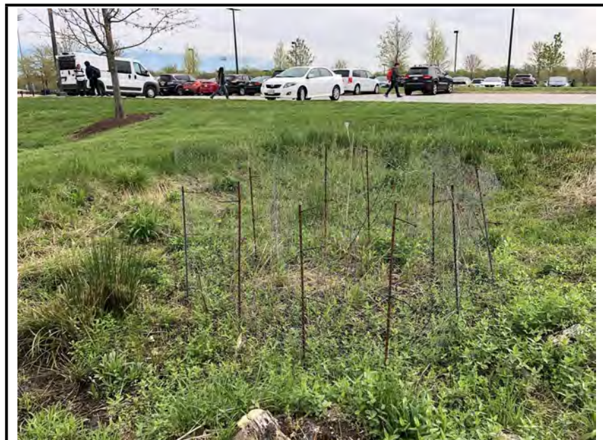
Photo #4: Chicken wire inside of facility filter area.
