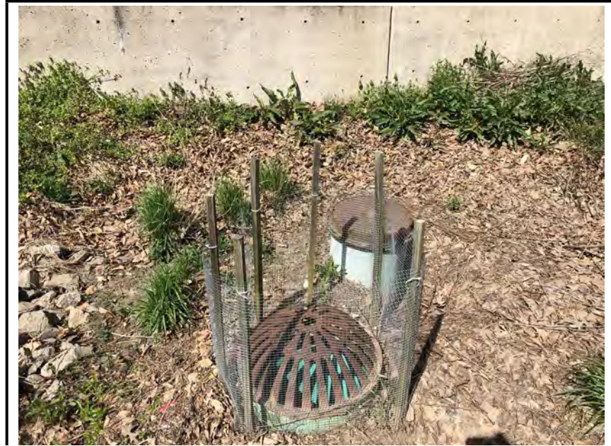
Photo #1: Riser outlet structure in facility.
