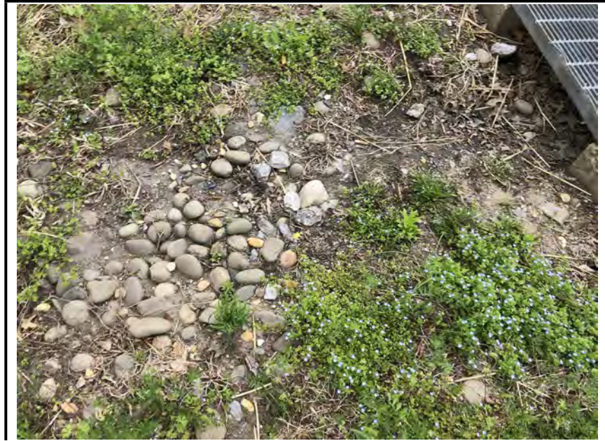
Photo #3: The inflow point of the facility.
