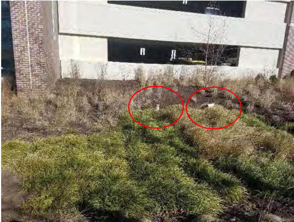
Inflow A - Pipe from Garage, Observation Well
