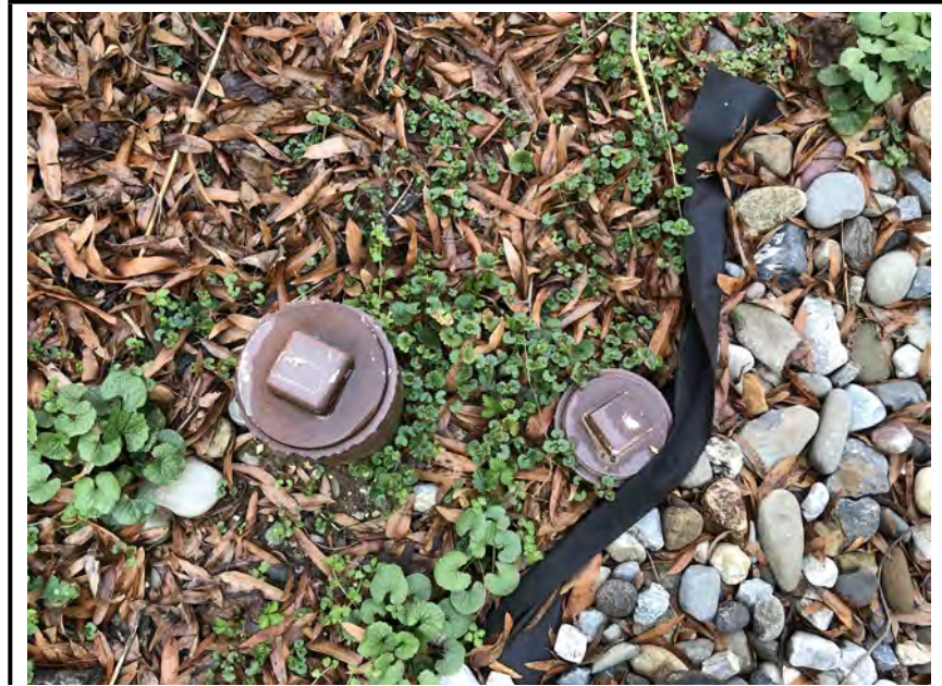
Photo #3: Exposed geotextile beneath stone inflow paths.
