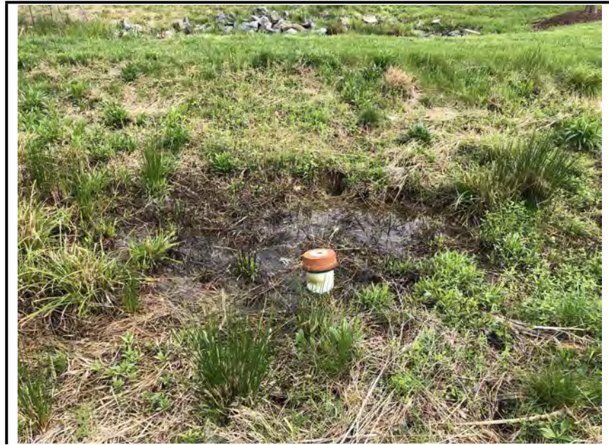
Photo #3: Ponding water around one of the cleanouts.
