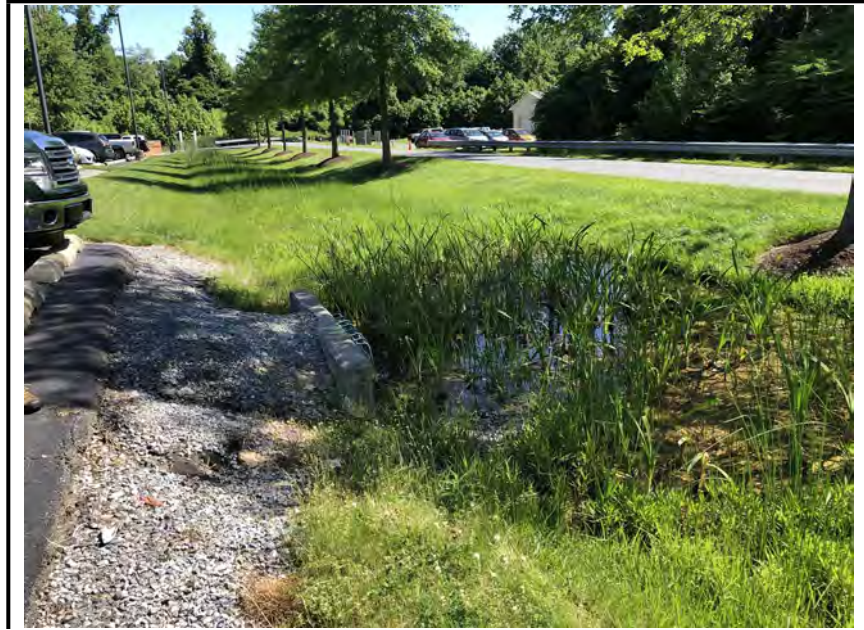
Photo #3: Pocket of standing water in the swale.
