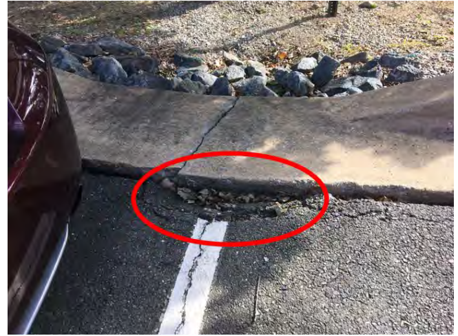
Figure 8 - Existing cracked asphalt
