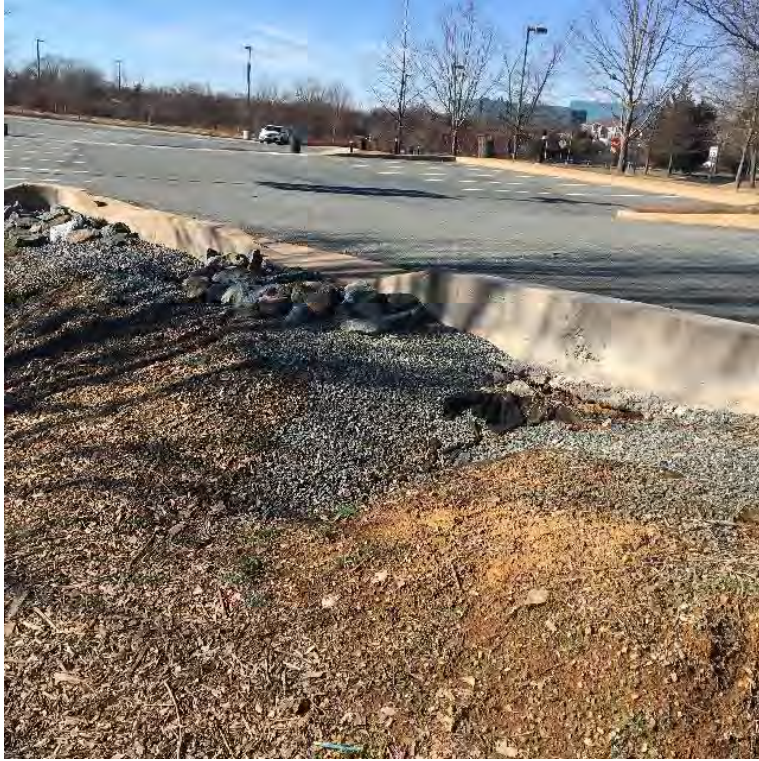
Gravel Curtain Drain Clogged
