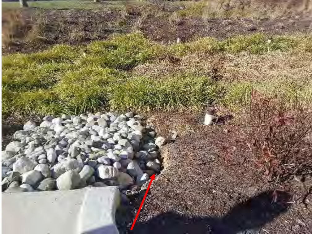
Erosion at Inflow A
