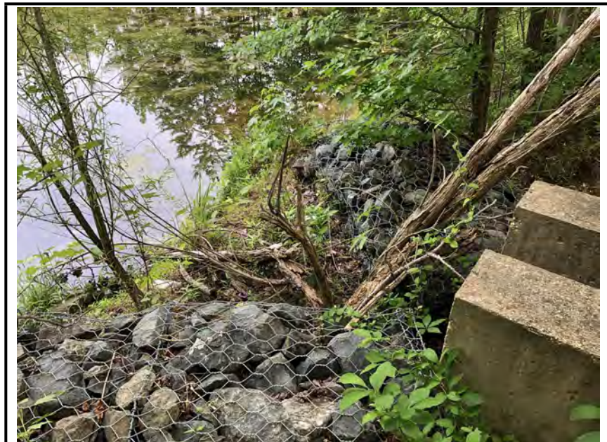
Photo #4: The v-notched weir that leads to the facility outfall.
