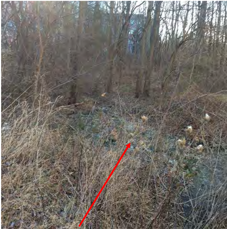
Embankment Blown Out at Control Structure
