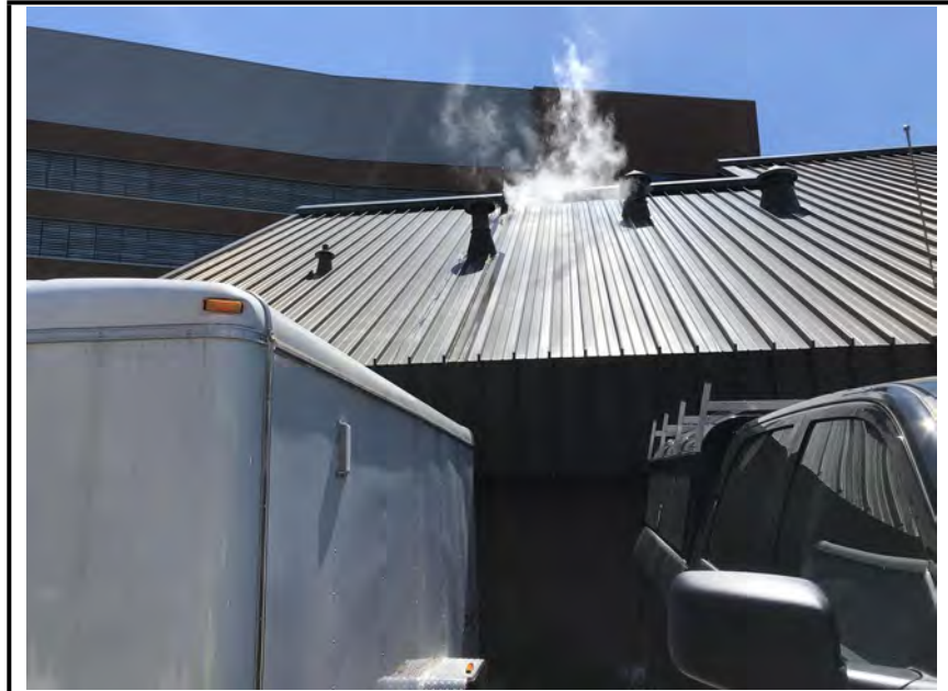
Photo #3: Steam from a vent that condenses on the roof and runs off onto the facility.
