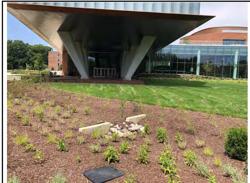
Photo #3: One of the weir walls. Notice the edges of the walls that do not tie not the sides of the swale.
