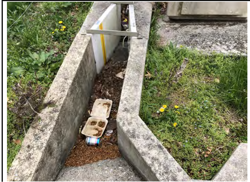
Photo #1: Trash and leaf debris clogging one of the concrete channels.
