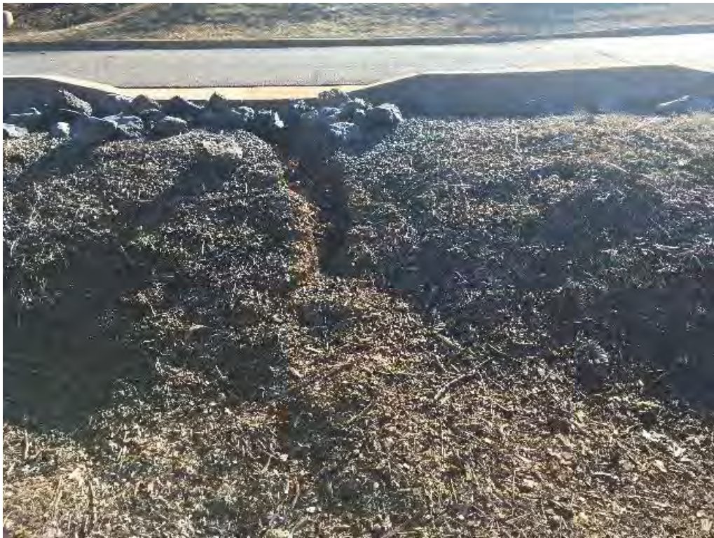
Erosion at Inflow A - Curb Cut - Facing South
