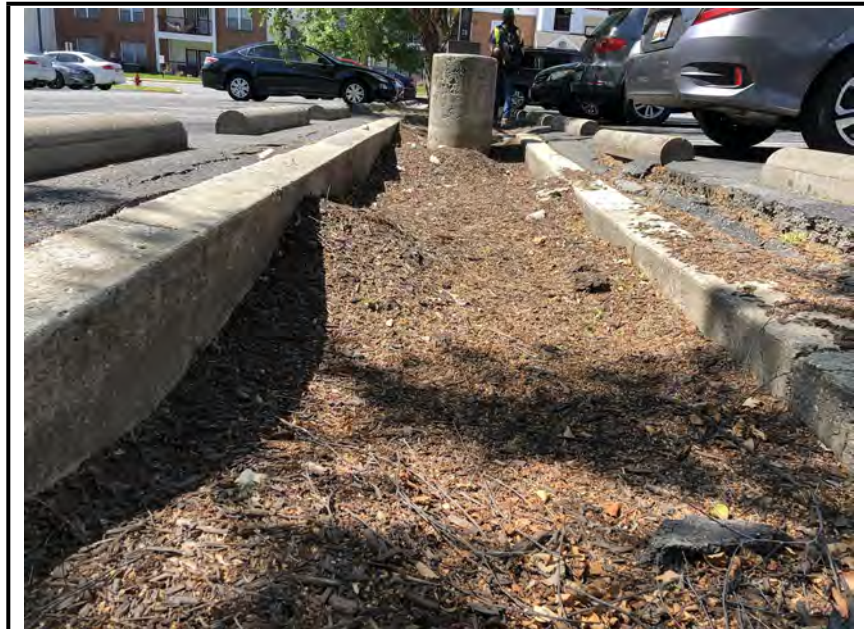
Photo #2: The uneven ground surface inside the facility.
