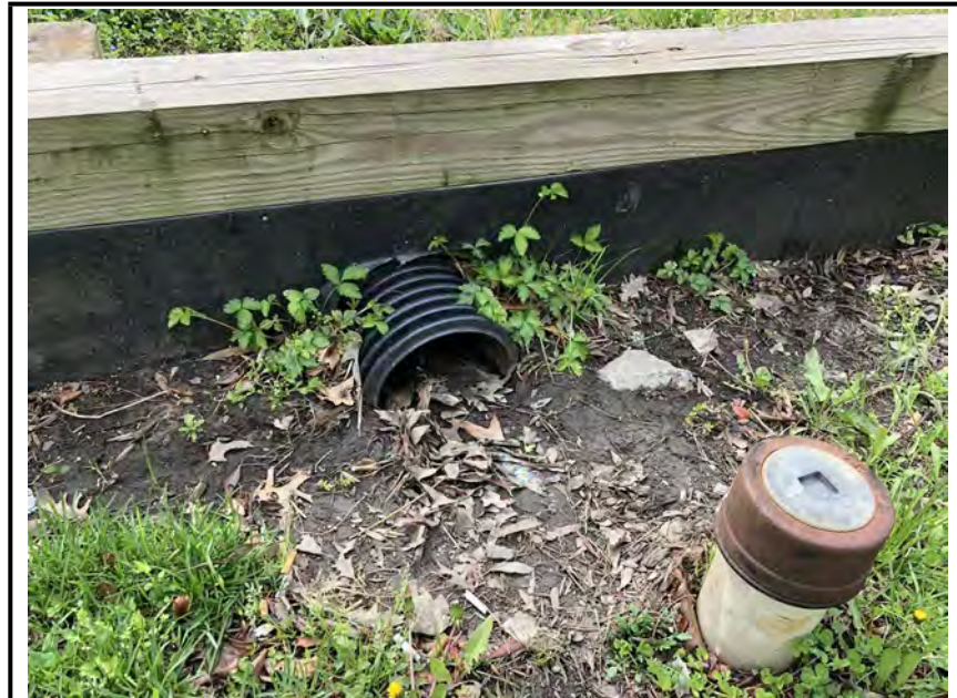
Photo #1: Clogged inflow pipe.
