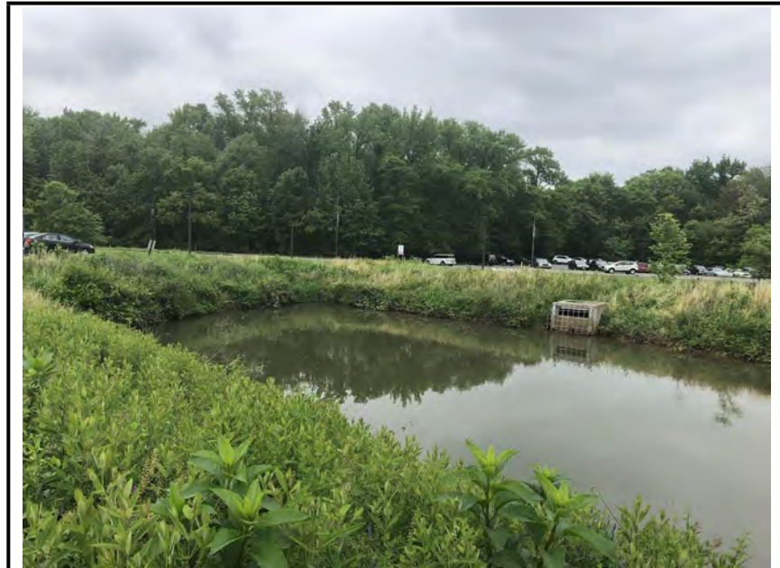
Photo #1: View into the facility. Outfall structure visible. Water is below the orifice.
