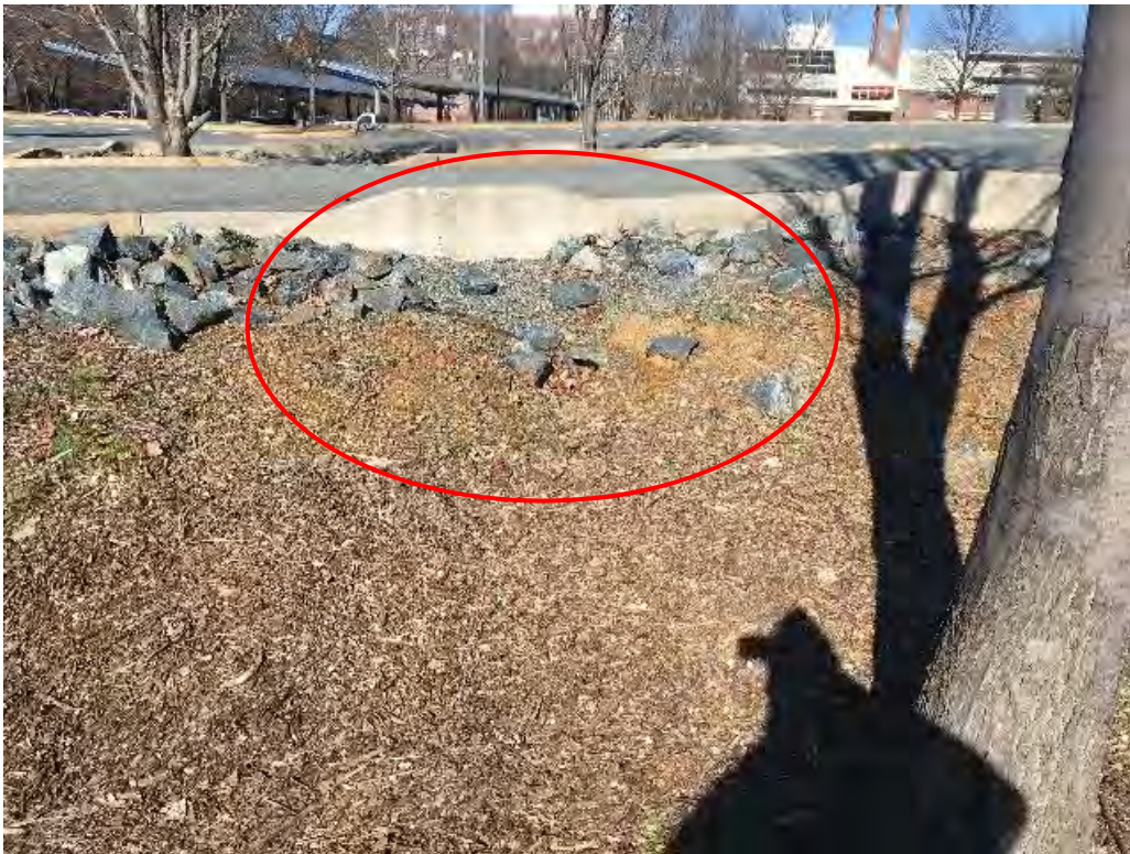
Erosion at Gravel Curtain - Facing North
