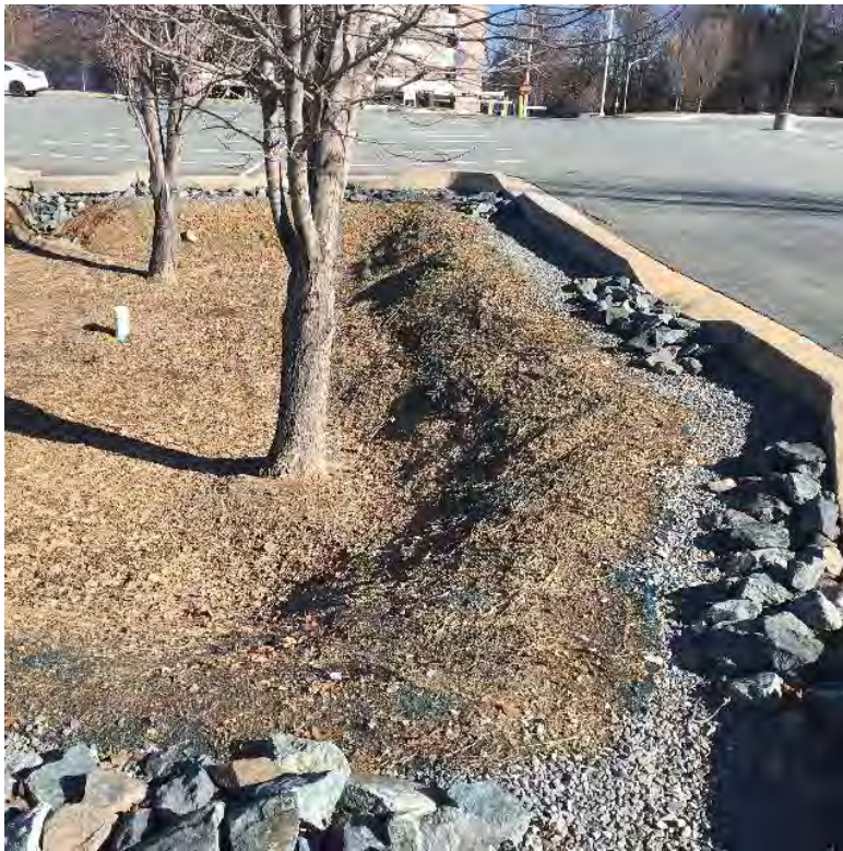
Steep Slope on BMP Embankment, Cleanout
