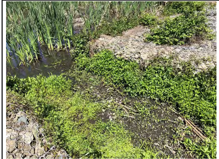
Photo #5: Sedimentation in the weir.
