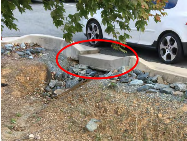
Figure 7 - Existing deteriorated curb and gutter
