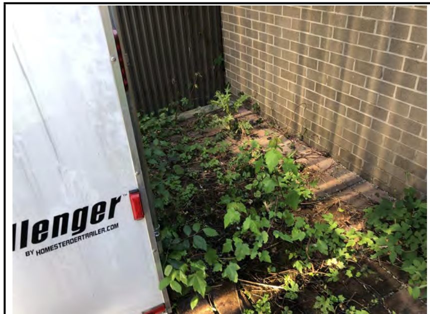
Photo #2: Vegetation growing from the facility surface.
