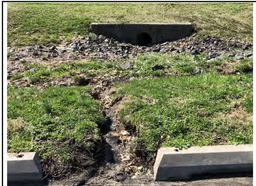
Photo #13: Erosional gullies downstream from the outlet culvert.
