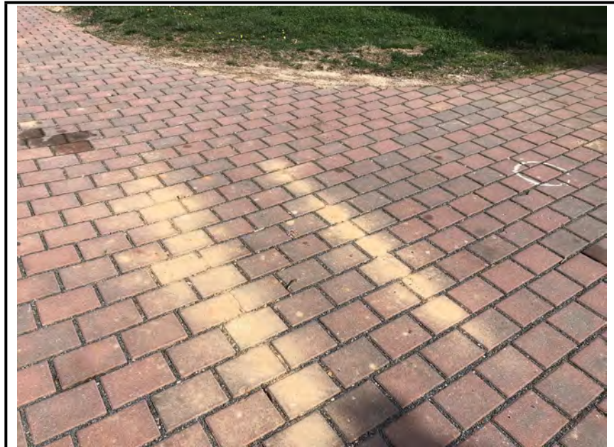
Photo #3: Dirt covering pavers.
