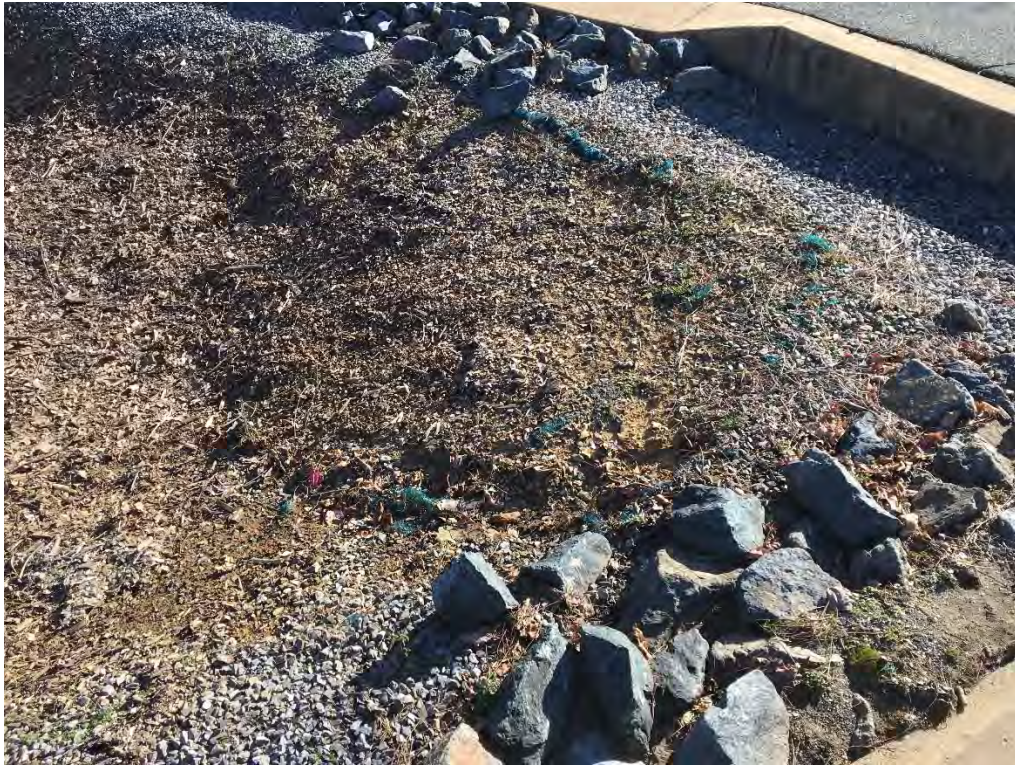
Sediment within Curtain Drain, Erosion at Curb Cut
