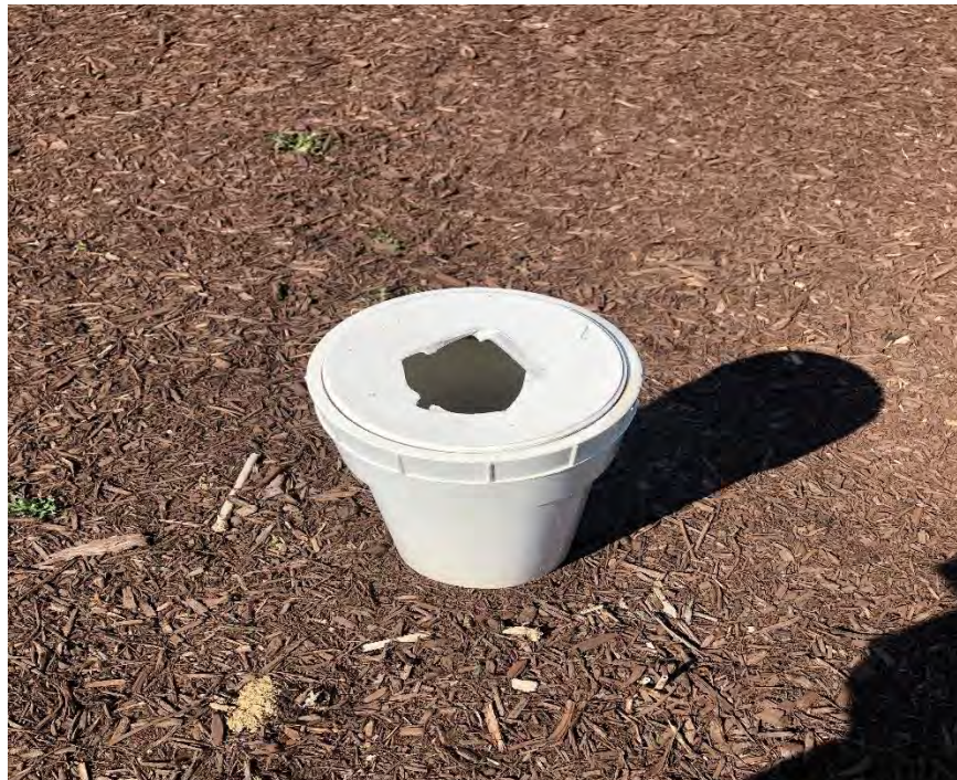
Photo #2: Broken cleanout inside the facility.
