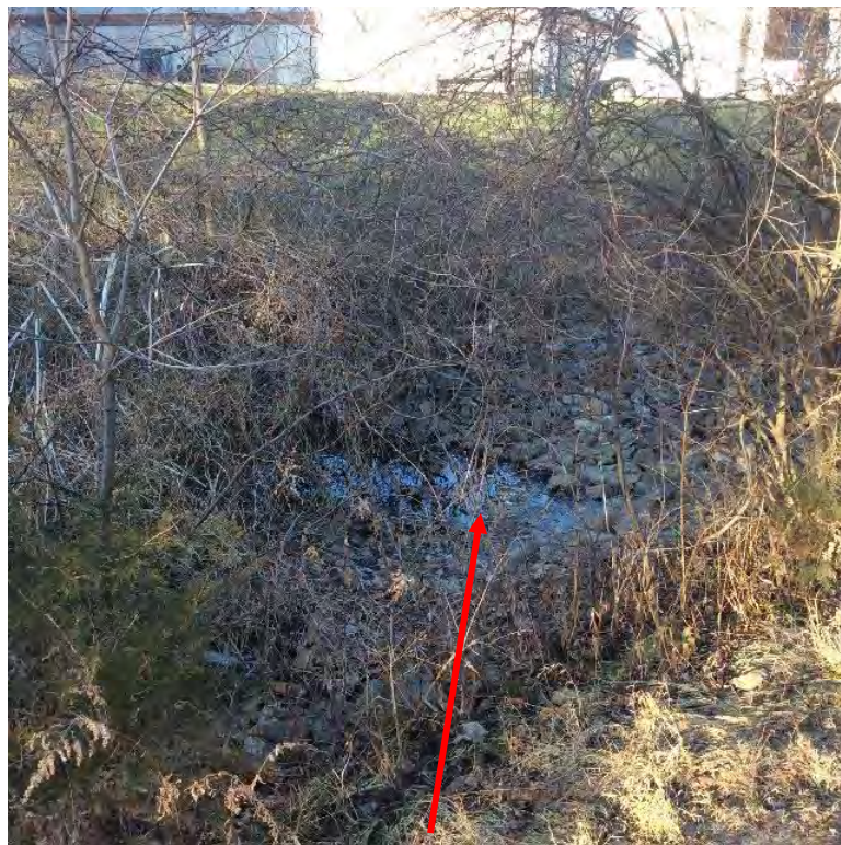
Inflow, Pipe Submerged
