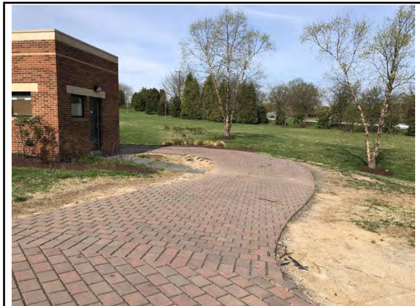
Photo #4: Eroded grass next to the pavers.
