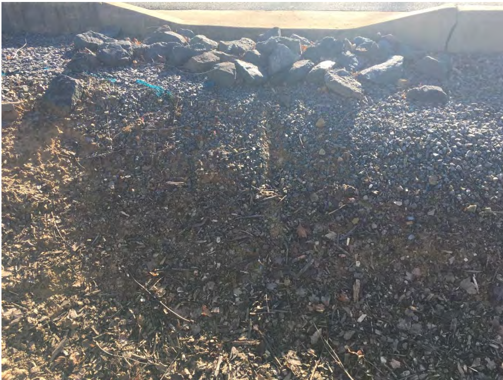
Erosion at inflow and embankment
