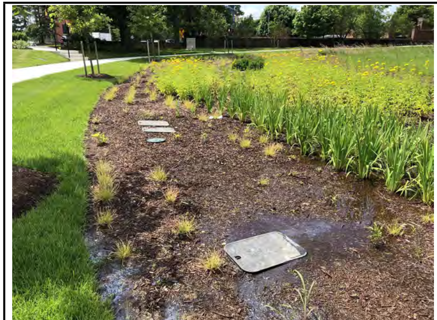
Photo #2: The effects of the backed-up irrigation system. Oil sheen is visible on water surface.
