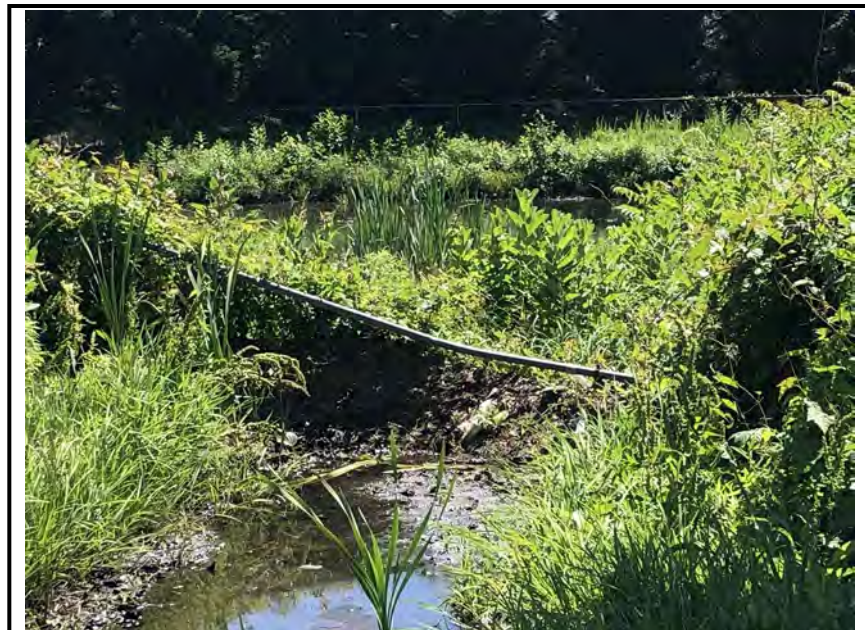
Photo #4: The section of collapsed and clogged fence in the inflow swale.
