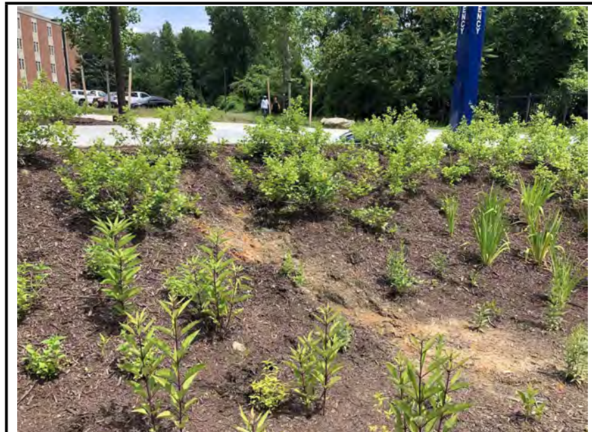
Photo #2: Erosion of the side slopes.
