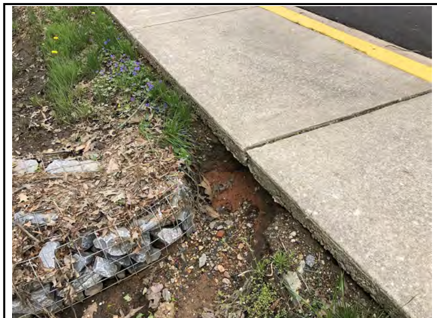
Photo #4: Gabion weir and undercut sidewalk.
