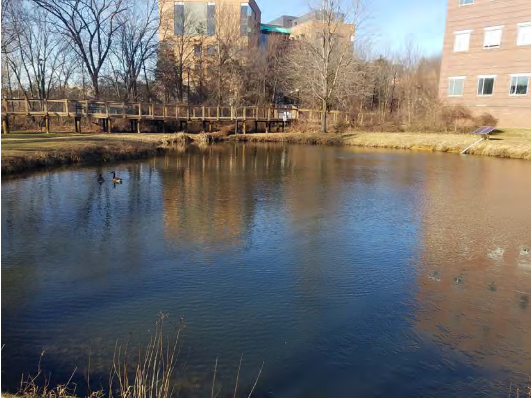
Upstream embankment, minor erosion
