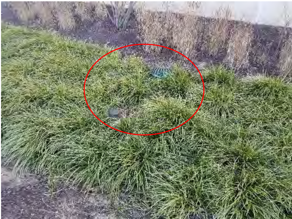
Overflow Device and Cleanout
