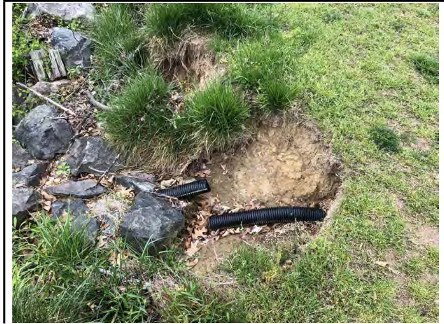
Photo #5: Broken pipe on edge of the filter area.
