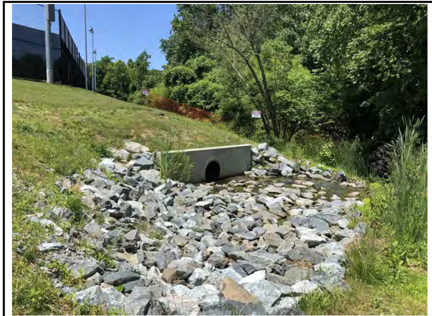
Photo #1: The inflow structure and pretreatment area.
