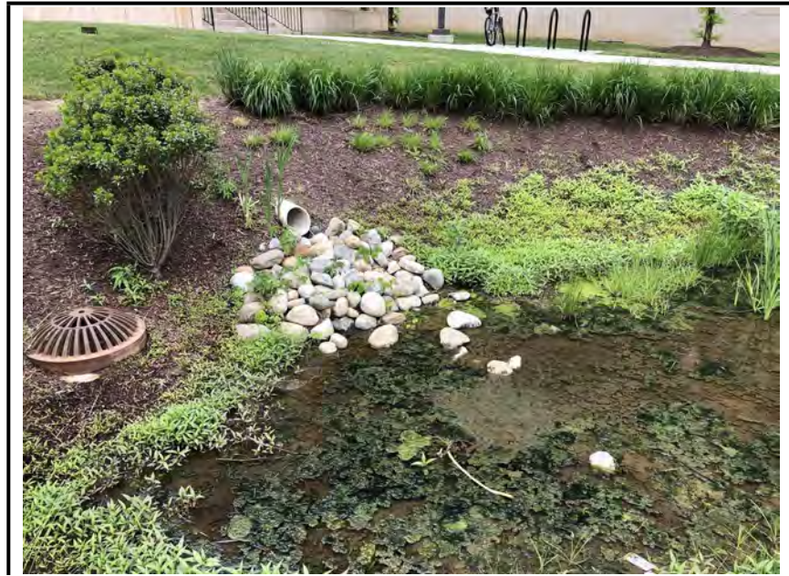
Photo #3: Algae and standing water next to the outflow structure.
