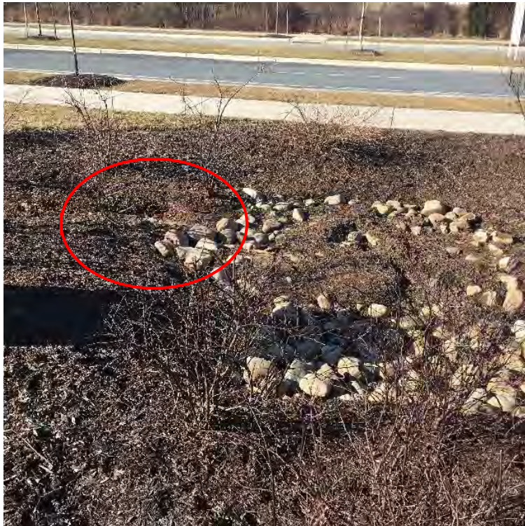
Inflow B - Flow from Sidewalk and planted area, Erosive flow into riprap
