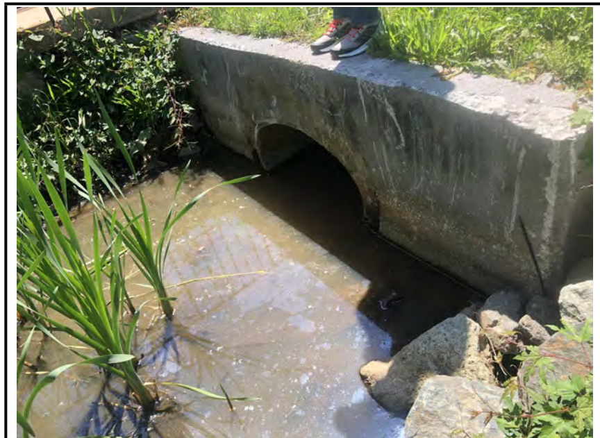
Photo #8: The inflow pipe with standing water.
