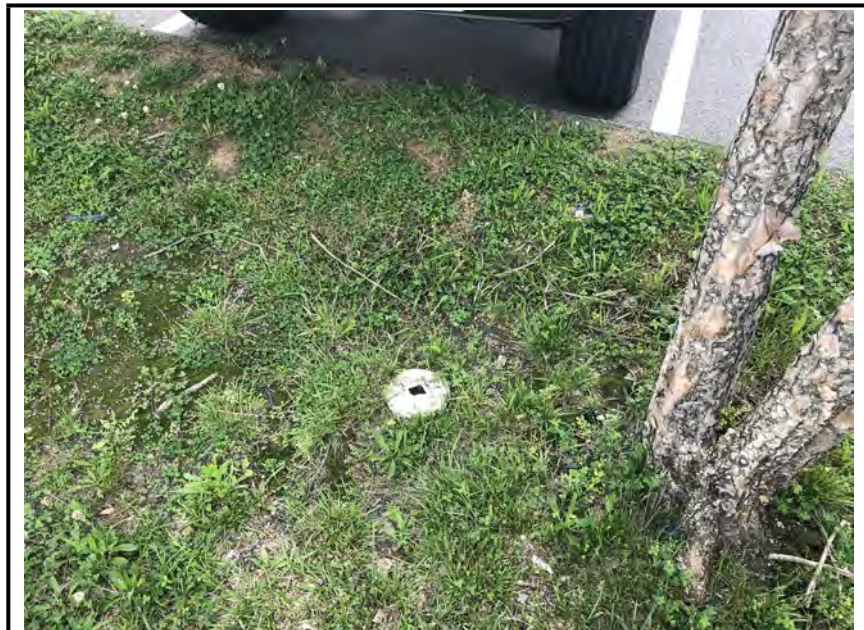
Photo #2: Broken cleanout.
