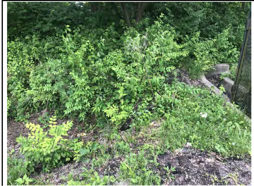
Photo #1: Overgrown vegetation in the filter area.
