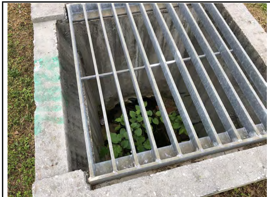
Photo #2: Vegetation growing inside the outfall structure.
