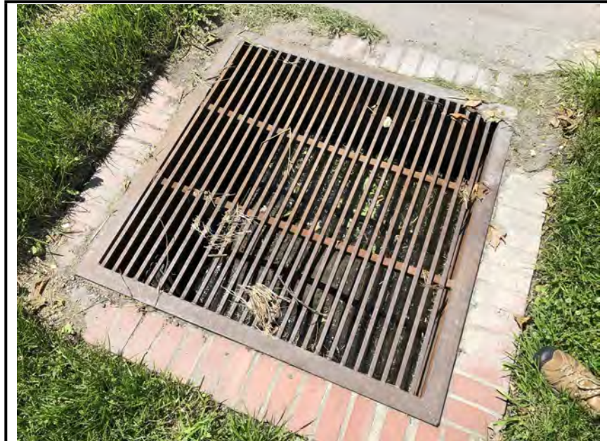
Photo #7: The aforementioned storm drain with manure inside.
