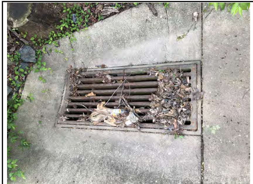
Photo #6: Outflow inlet clogged with leaves and trash.
