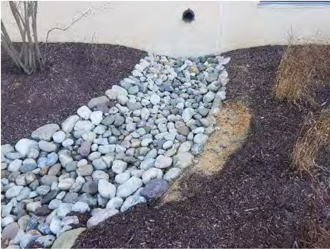
Inflow B, East - Erosion at inflow
