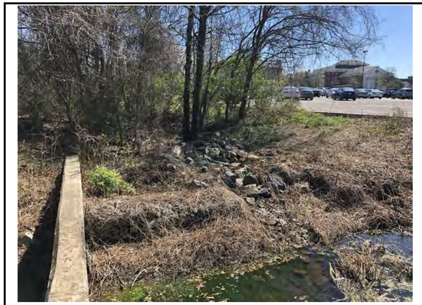
Photo #1: Flowsplitter, algae, vines, and debris present.
