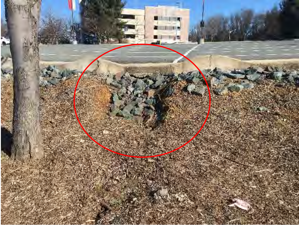
Erosion at Inflow B - Curb Cut - Facing West
