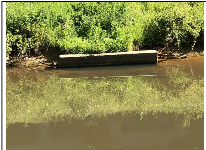
Photo #4: The unidentifiable submerged headwall.
