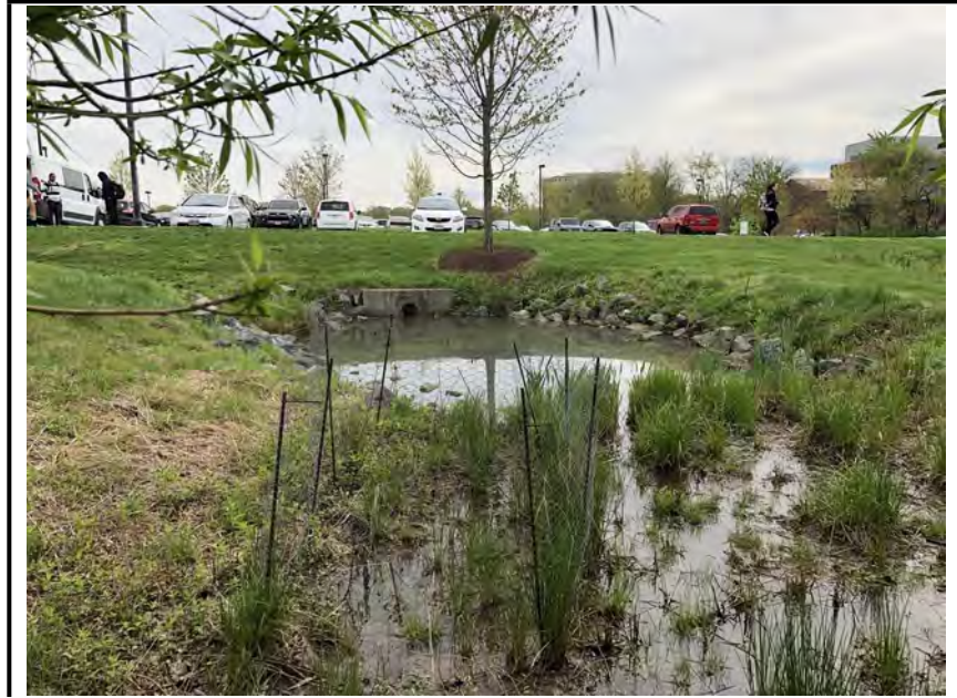
Photo #5: Forebay pretreatment area.
