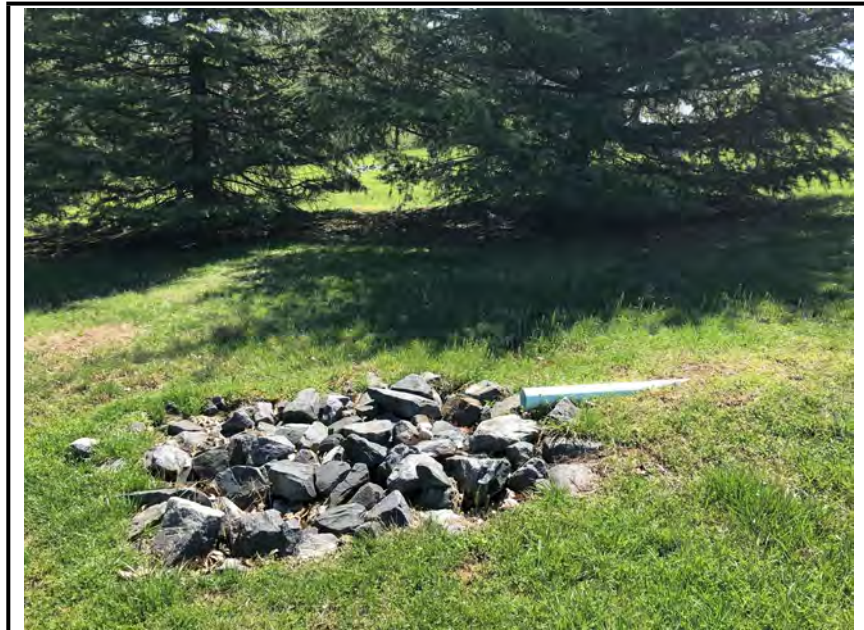
Photo #5: One of the exposed underdrains.
