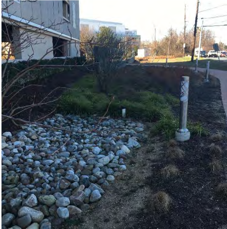
Overall - Facing North, Minor Erosion at Riprap
