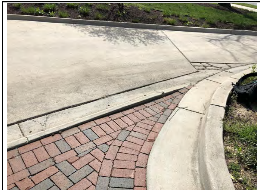
Photo #2: Curb is not flush to the pavers.
