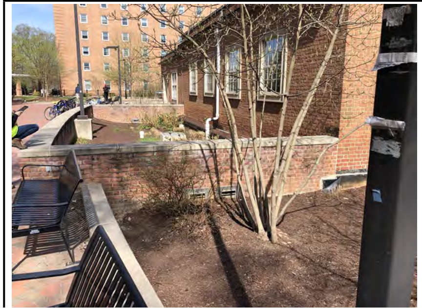
Photo #3: Wall openings that lead from the forebay into the filter area.
