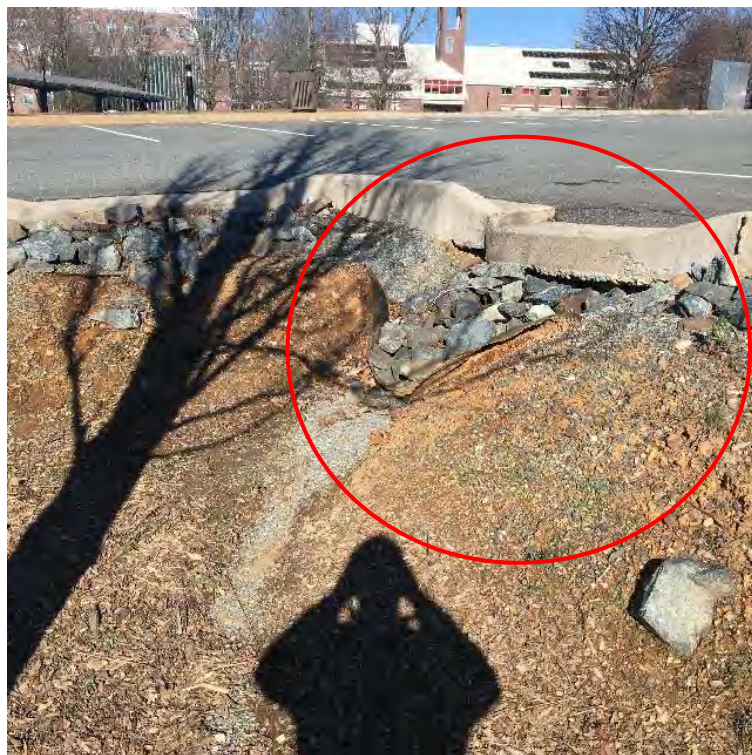
Inflow - Curb Cut, Facing West, Curb Damaged and Undermined
