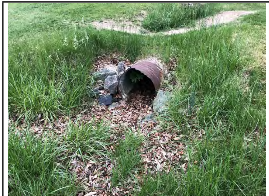
Photo #4: Erosion above inflow pipe.
