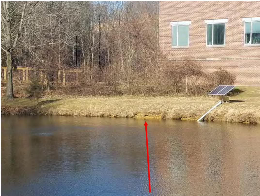
Erosion at embankment toe
