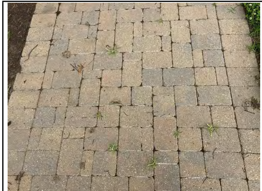
Photo #2: Vegetation growing in cracks in the pavers.
