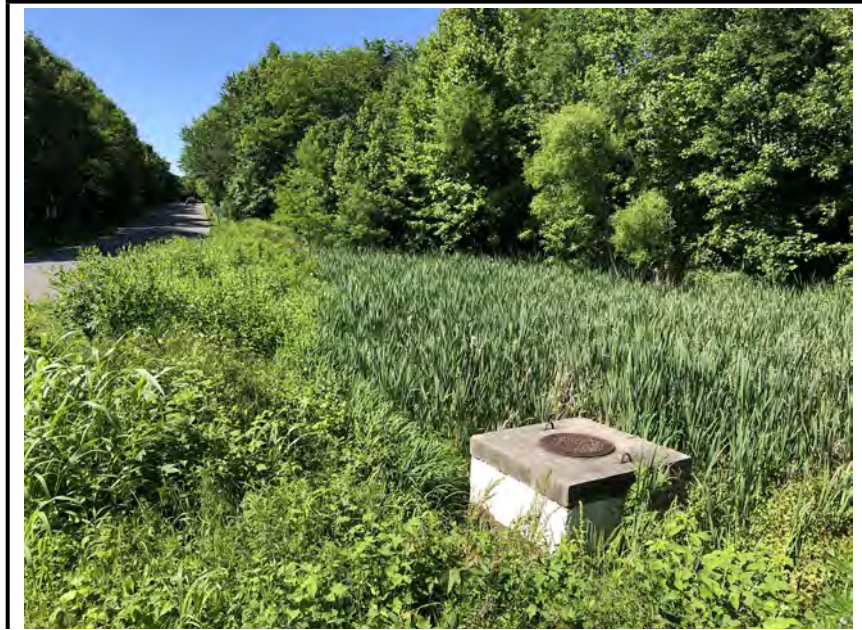
Photo #1: View into the facility. Filter area is completely covered with cattails.
