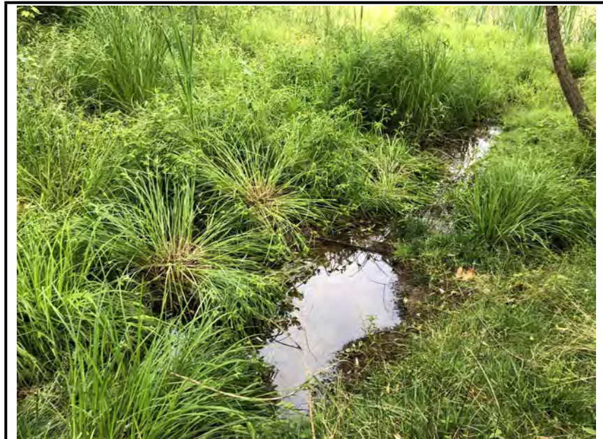
Photo #6: Inflow channel that lacks riprap to protect from erosion.
