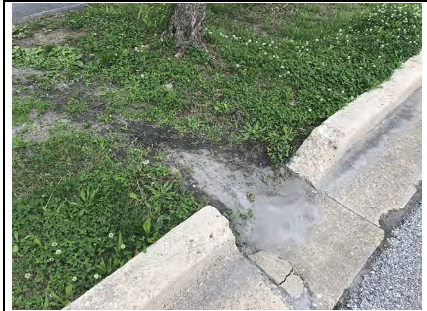
Photo #1: Eroded curb cut.
