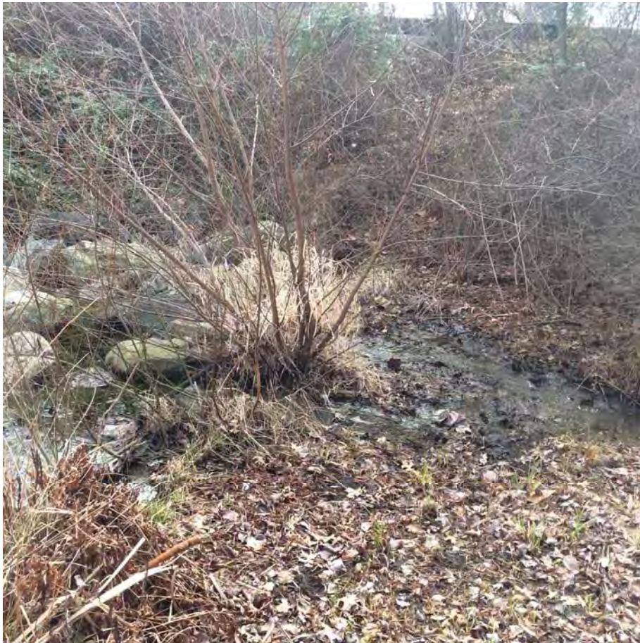
Tree Growth at Outflow of Emergency Spillway
