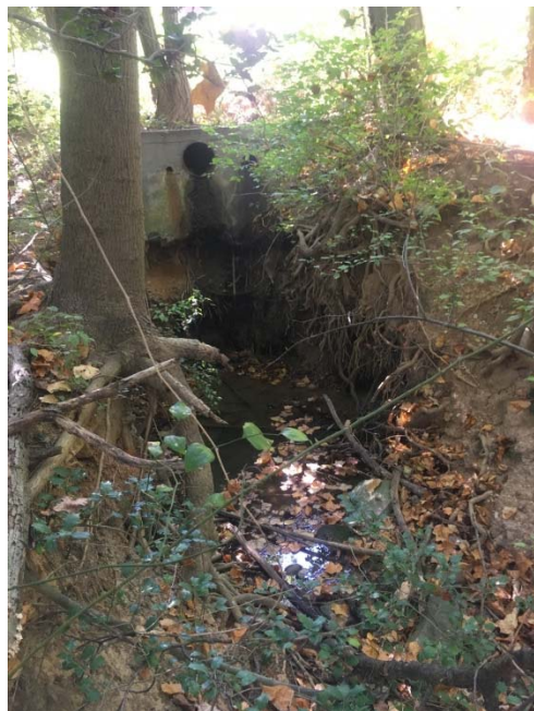
Figure 4. OF 42 Tree growth and erosion damage
